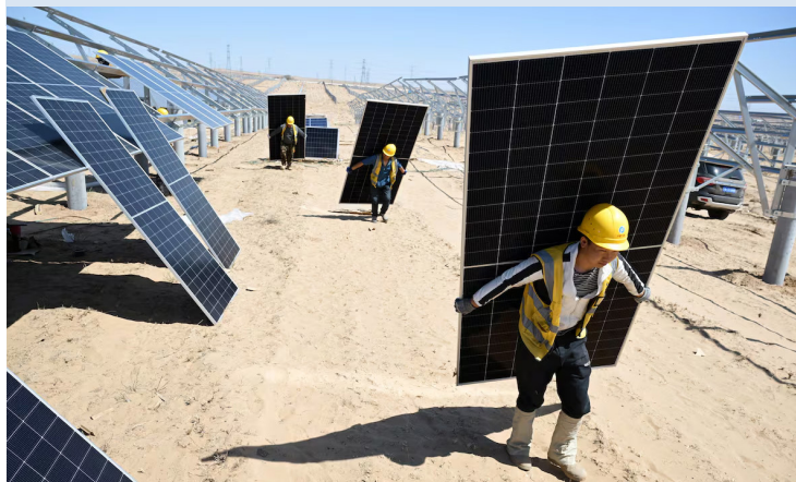
Workers install a solar park in the Ningxia Autonomous Region, China. Photo: VCG via Getty Images.
